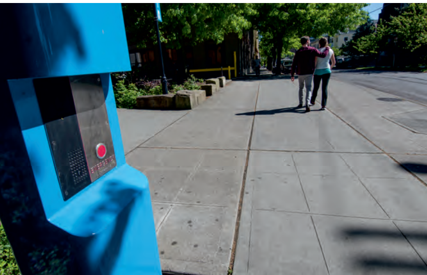
A Talkaphone WEBS-MT/R tower housing a VOIP-600E call station looks over Seattle Central College campus (photo credit: Bethany Baker/Seattle Central College)
